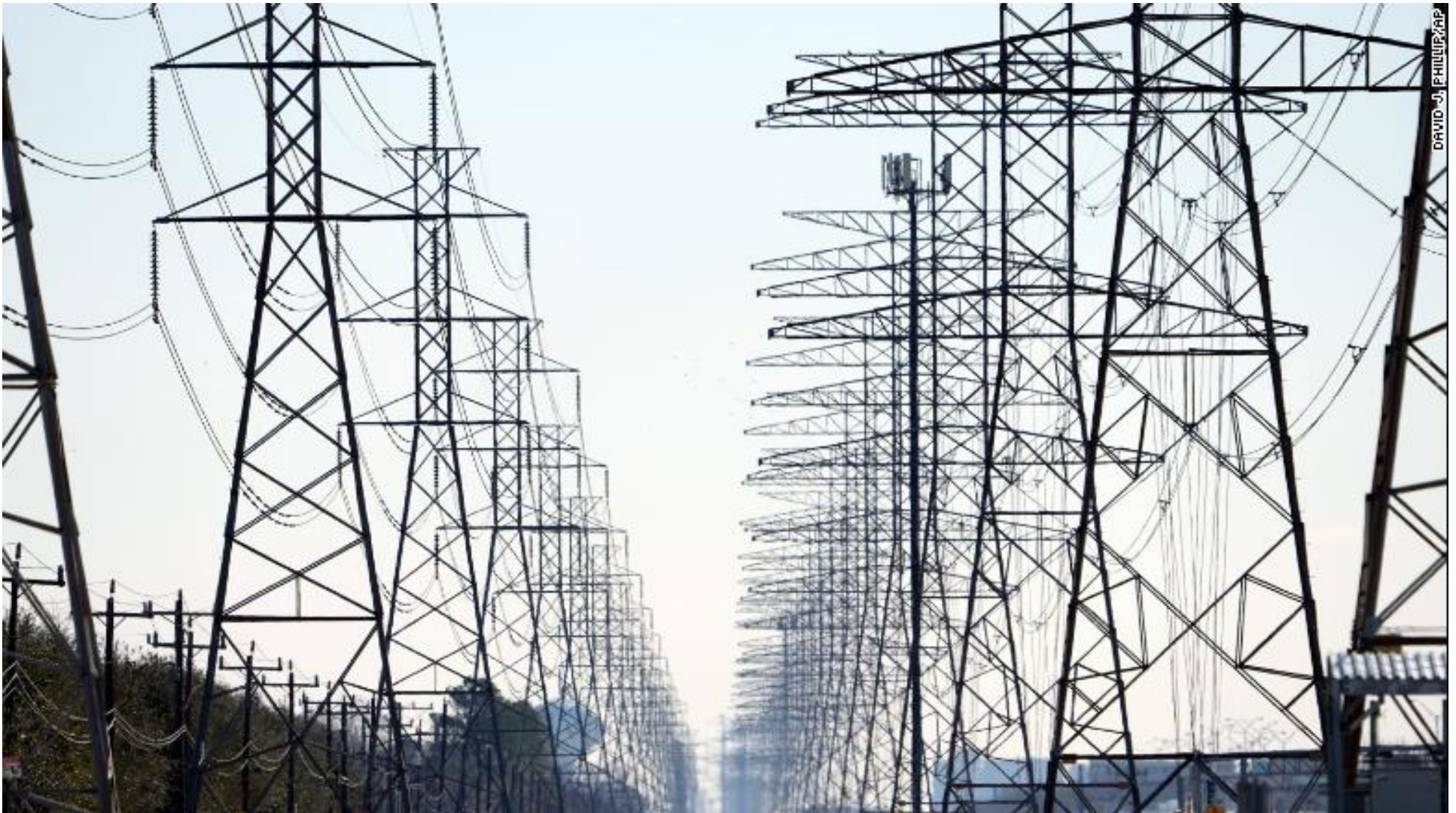
Power lines in Houston, Texas on Tuesday, February 16, 2021.
