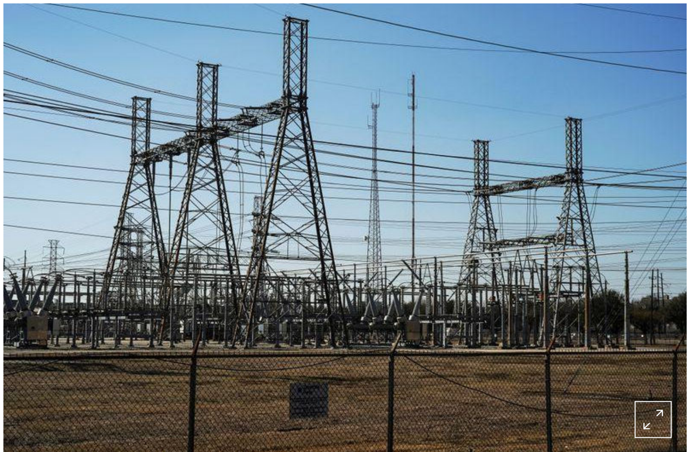
FILE PHOTO: An electrical substation is seen after winter weather caused electricity blackouts in Houston, Texas, U.S. February 20, 2021. REUTERS/Go Nakamura
